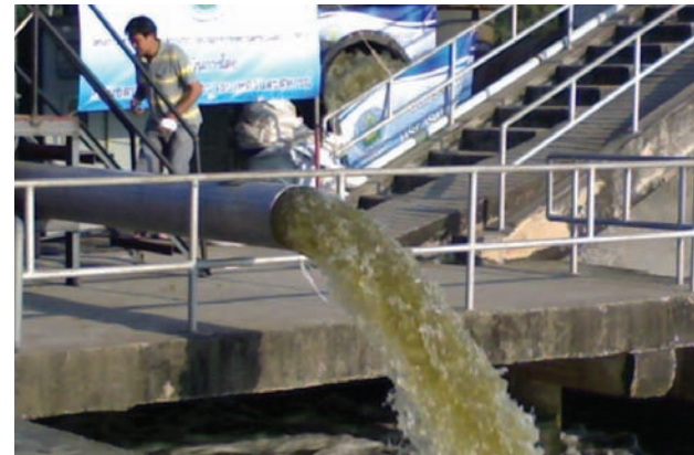
CORNELL'S 14NHG-RP-F18DB DEWATERS MILLIONS OF GALLONS DURING FLOODING
