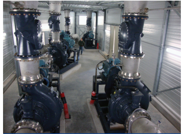
EXPANSION OF BRUSSELS SEWAGE PLANT WITH SIX CORNELL MODEL 18NHFL-RP-F20 PUMPS, EACH PUMPING 2500M3 PER HOUR
